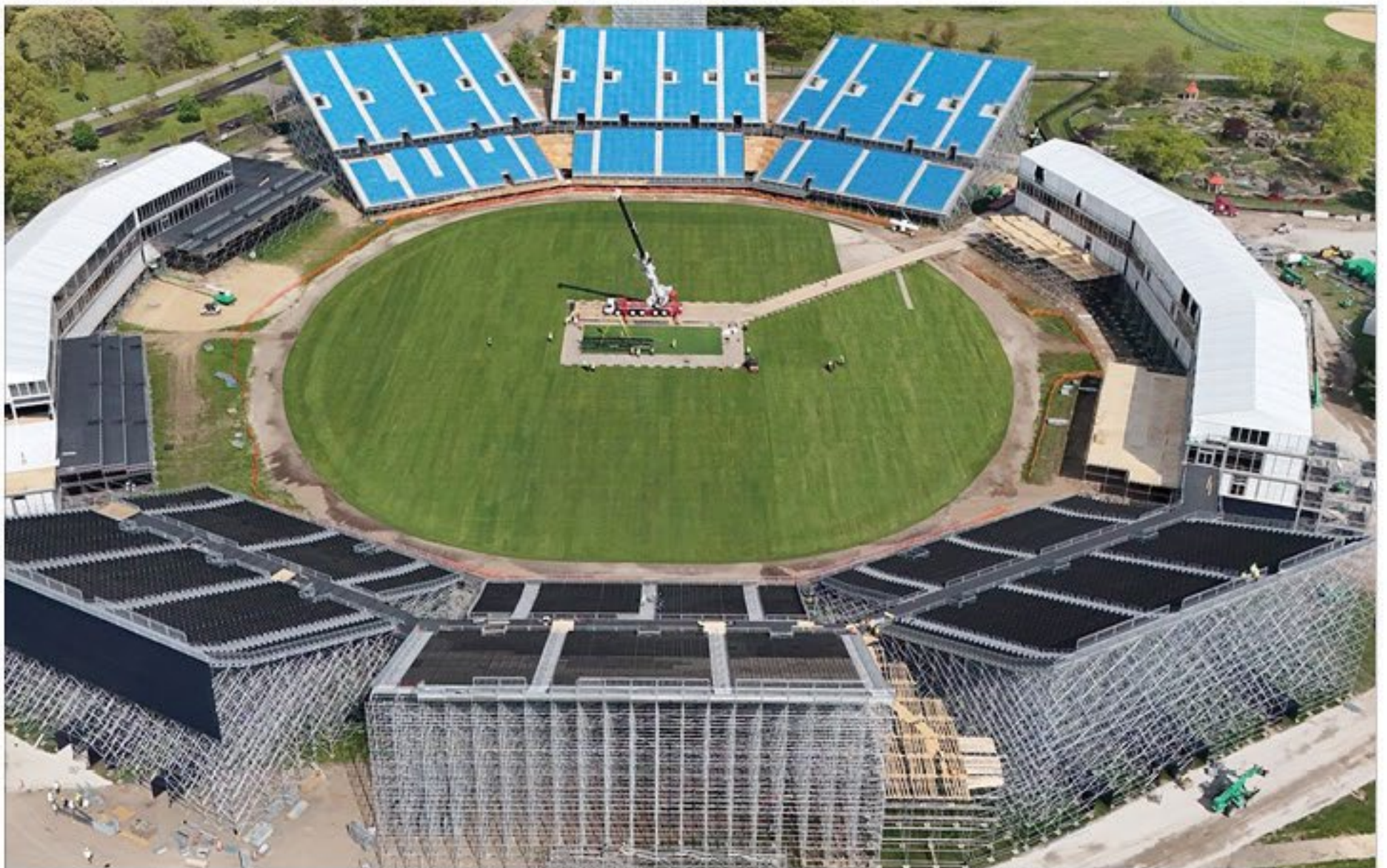
The project involved erecting a fresh stadium in five months, with drop-in pitches transported from Florida by land to New York
